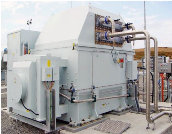
Synchronous condenser unit
