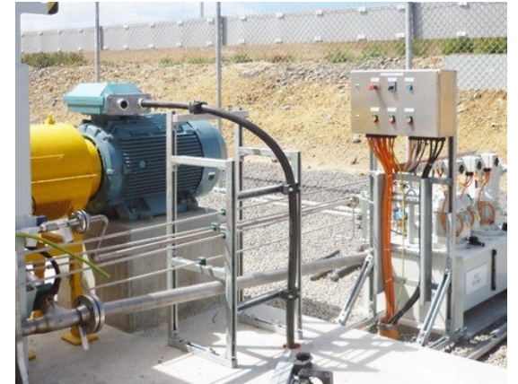
Pony motor Lube oil tank unit
