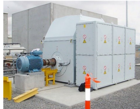
Main terminal box
