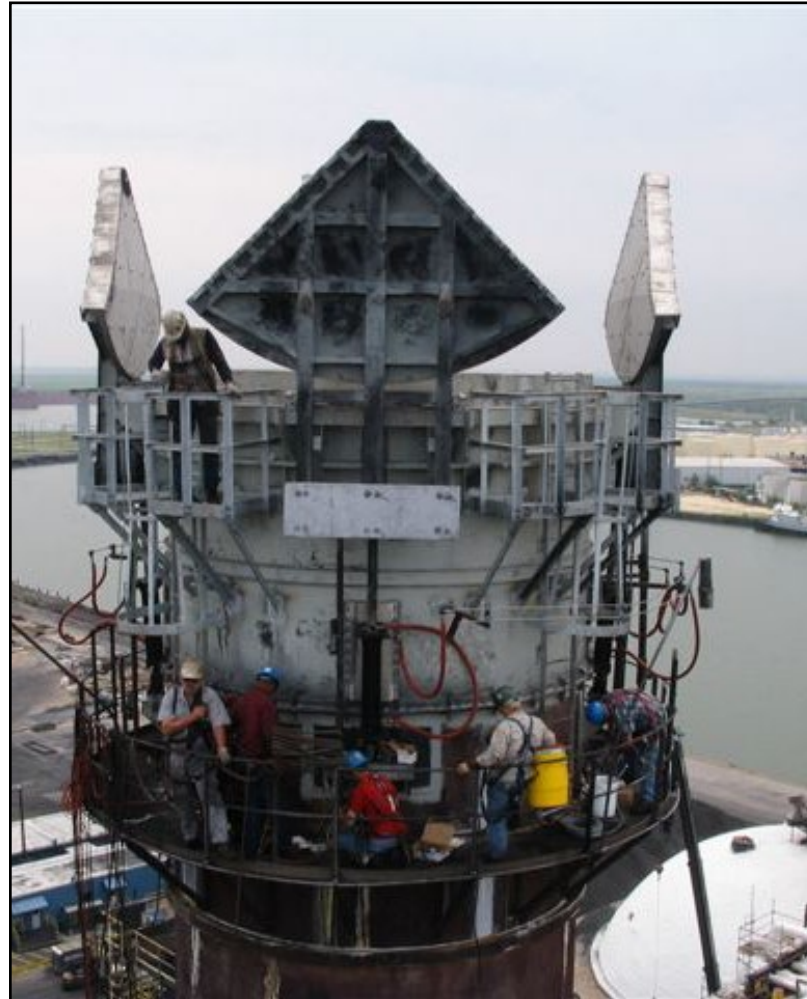
Kiln Stack “Cap” Exhaust Diverter
