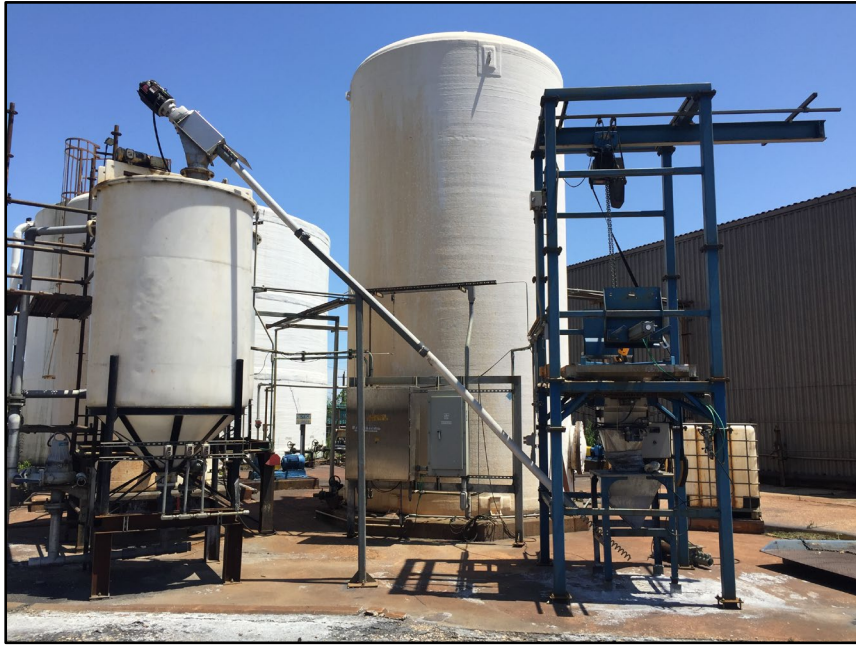
On-site Magnesium Hydroxide Mixing System
