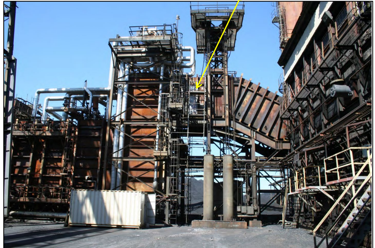
Injection point in boiler inlet duct
