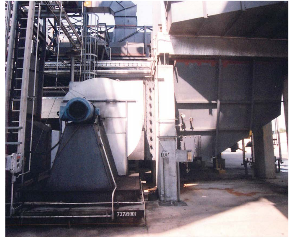
Induced Draft Fan
