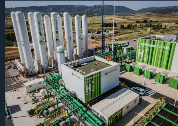
20 MW KOH plant: 5,000,000 cm 2 200,000x test cell
